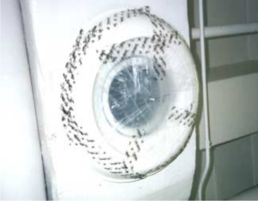
Figure 3. Sealed diffuser in Building LS-2
