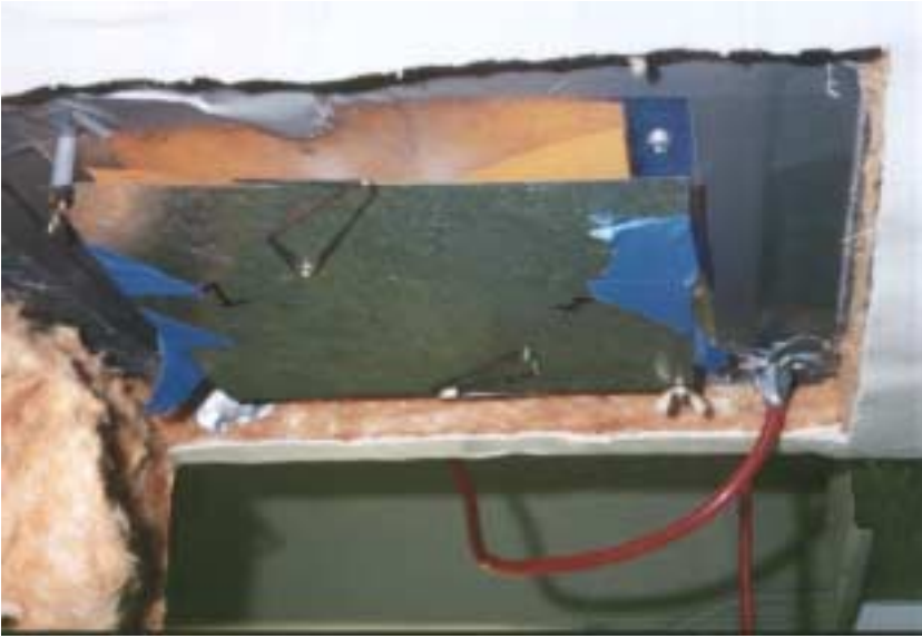
Figure 6. Impaction plate installed in Building LS-2
